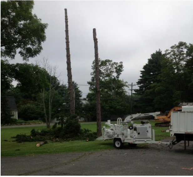
Several trees have been removed to make way for the new building foundation
